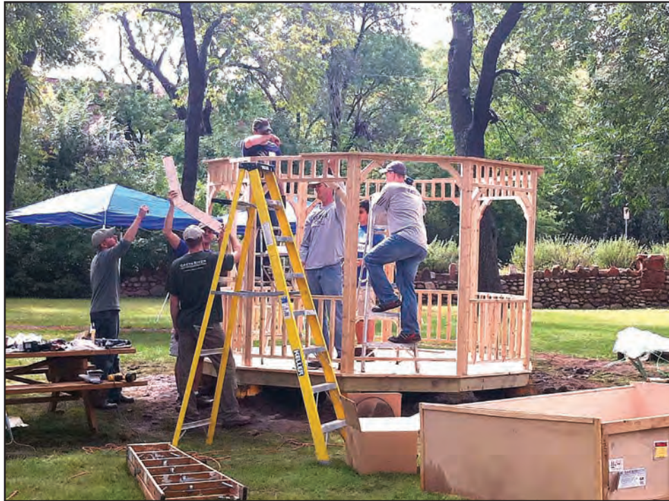
RLH employees work with Family Life Services on site to install a new gazebo.
